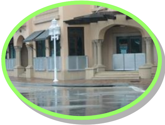
Closures applied to windows and doors during a storm event to keep floodwater from entering.
