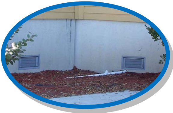
Vents allow floodwaters to enter into the home.
