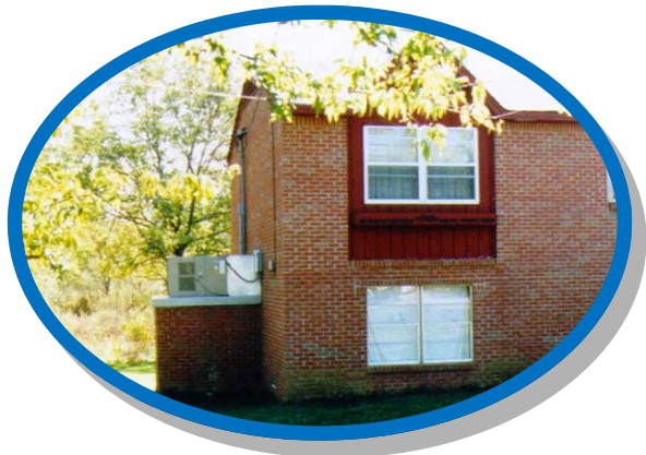
Utilities elevated above the flood elevation.
