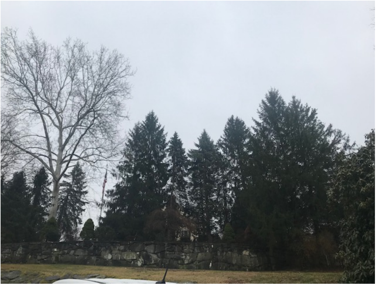
Large trees growing above the retaining wall.
